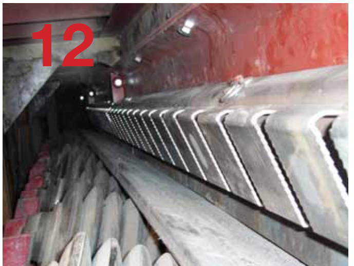
EZ-SKIRT® 5-foot hangers pinned on to each door. Only skirting left to quickly insert.
