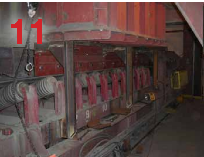
15-foot Pre-assembled section in place. This side installed with all support structure pre-attached.
